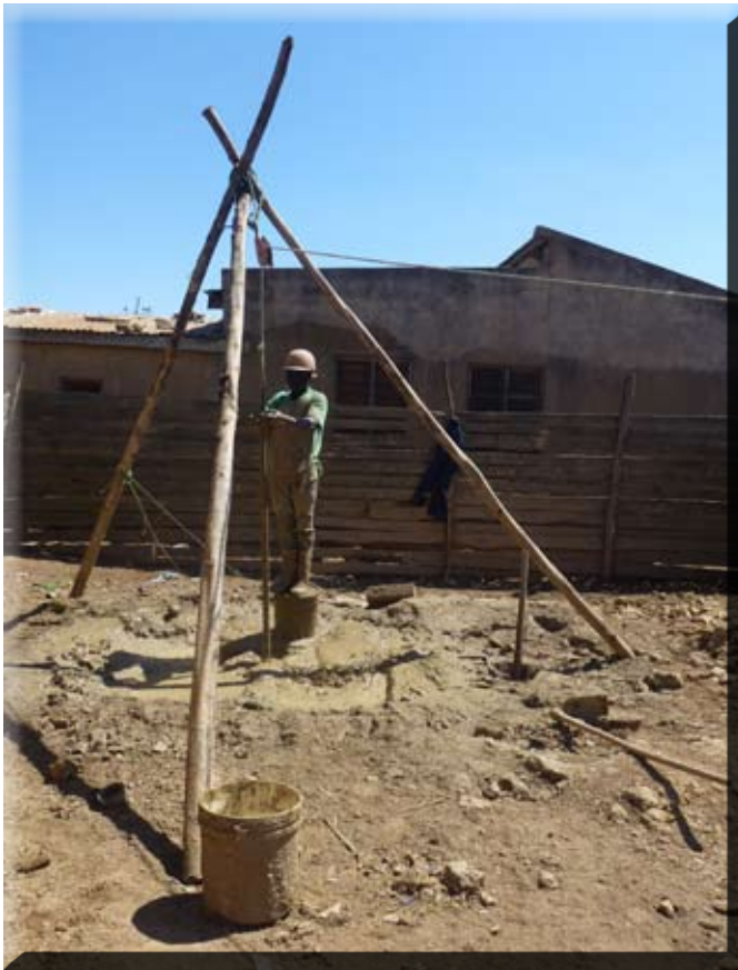
Mr. Edmsy Kitemi one of SHIPO Trainees spotted drilling in Makambako Town by using SHIPO drilling method .
